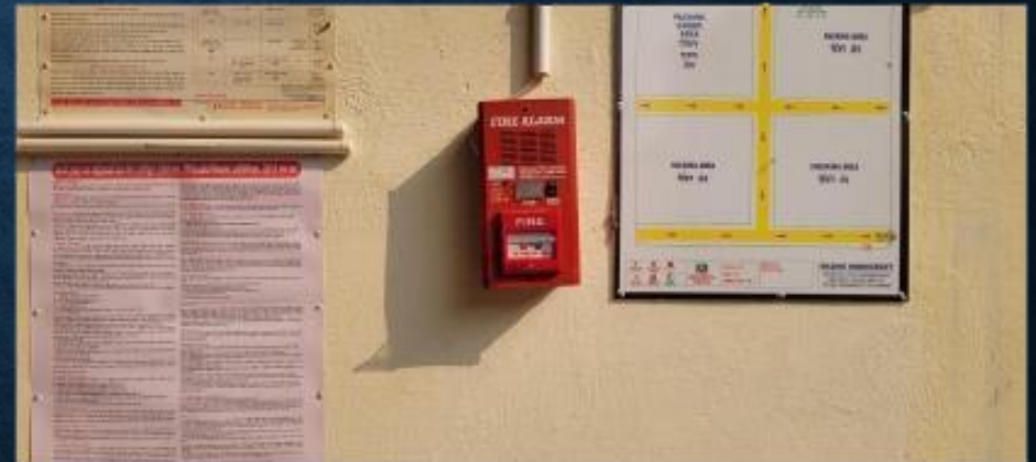
NC- No Instruction for the use of Fire Alarm
